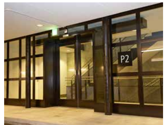
Automatic fire-protection door, multi-storey car park
