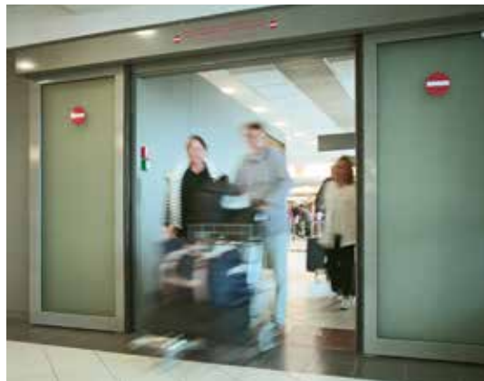
Automatic fire protection door, baggage claim, LYS
